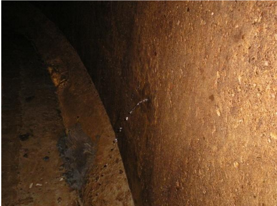
Leaking and deteriorating main reservoir in San Ignacio
