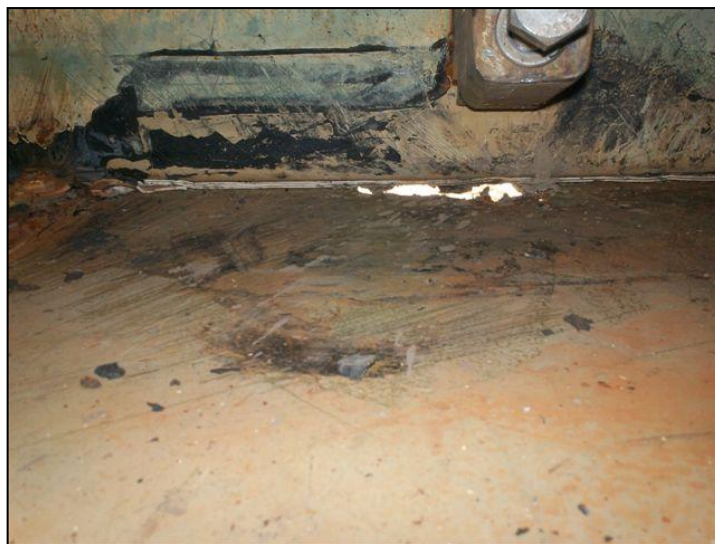
Leaks at the Southside Reservoir - Belize City
