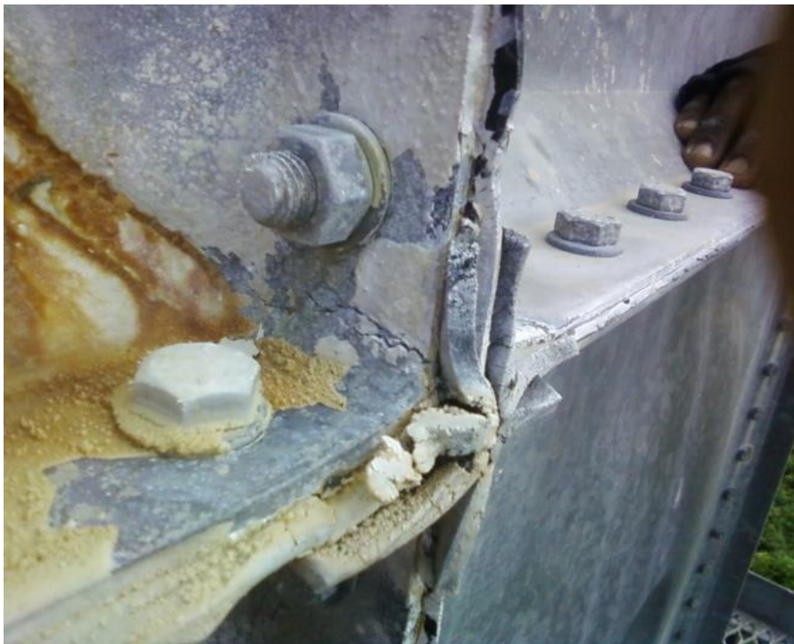
Leaking and deteriorating reservoir in Corozal
